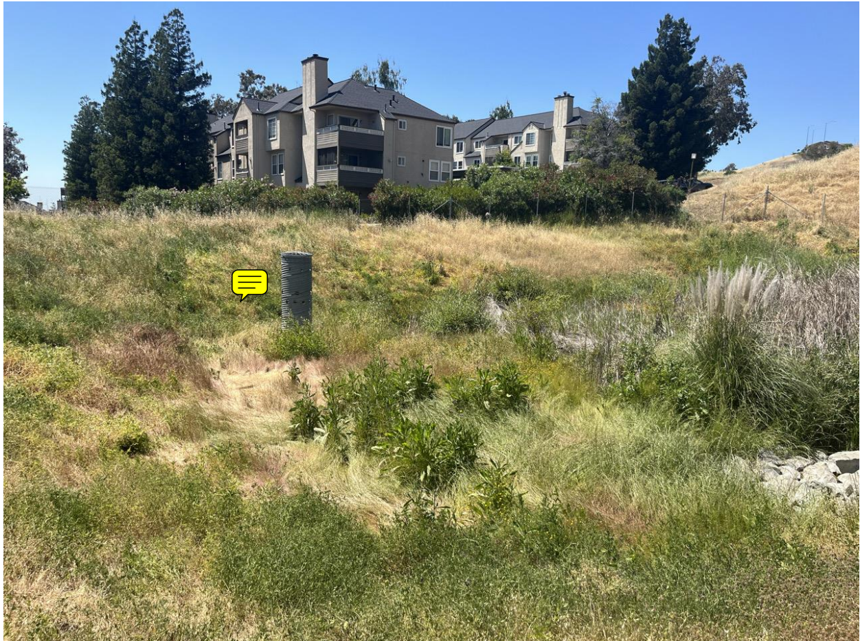
PHOTO 3: Site Condition B – Alquire Water Retention/Detention Facility with Overgrown Vegetation
