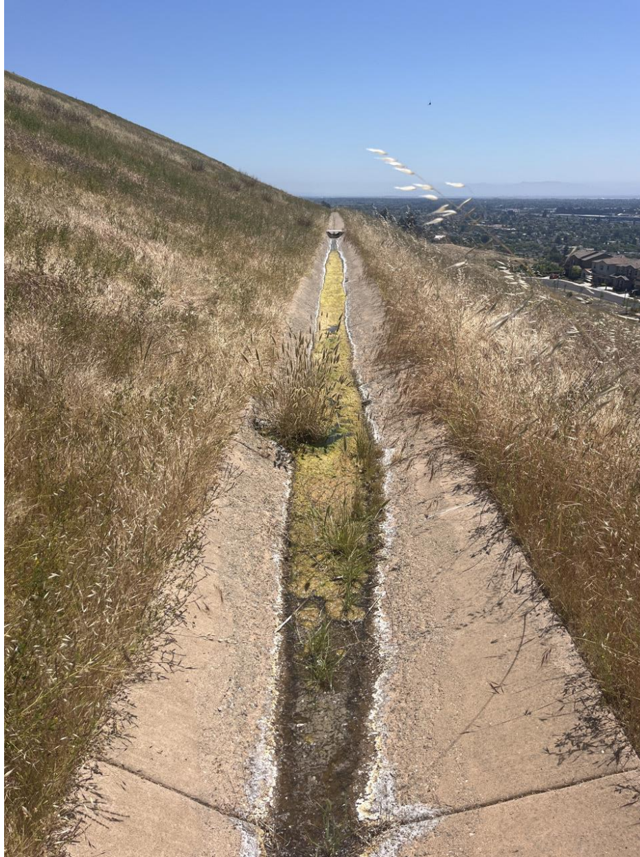
PHOTO 4: Site Condition C – Standing Water and Overgrowth around Subdrain SD-07 Outlet.
